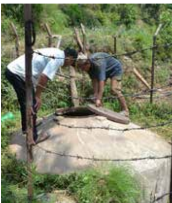
Both the reservoir and water tap (photo at right) were reused from the old system.
