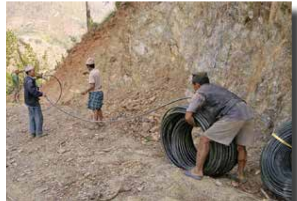
Once the trench was dug, they laid 3,000 feet of high-density pipe to connect the spring with the reservoir tank.
